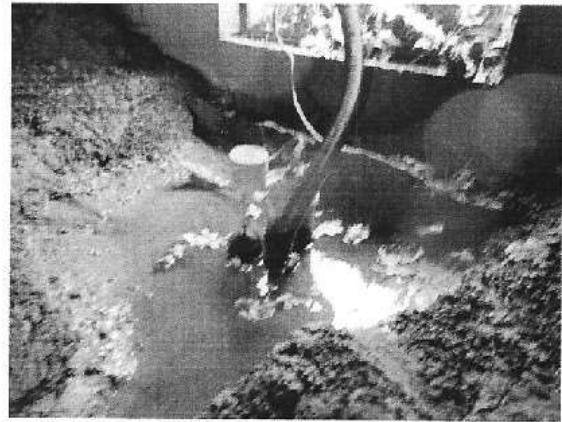
Sump pump in mud at crawl entrance.
