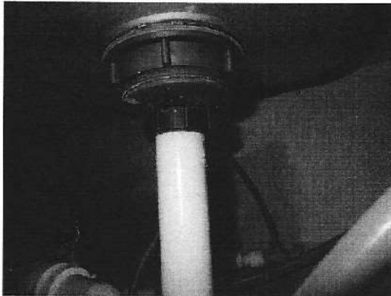
Right side of kitchen sink drain is leaking.
