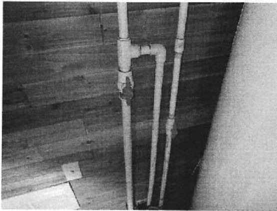
Main water shutoff at east wall utility room.
